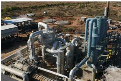
Sulphuric Acid Plant (SAP)
